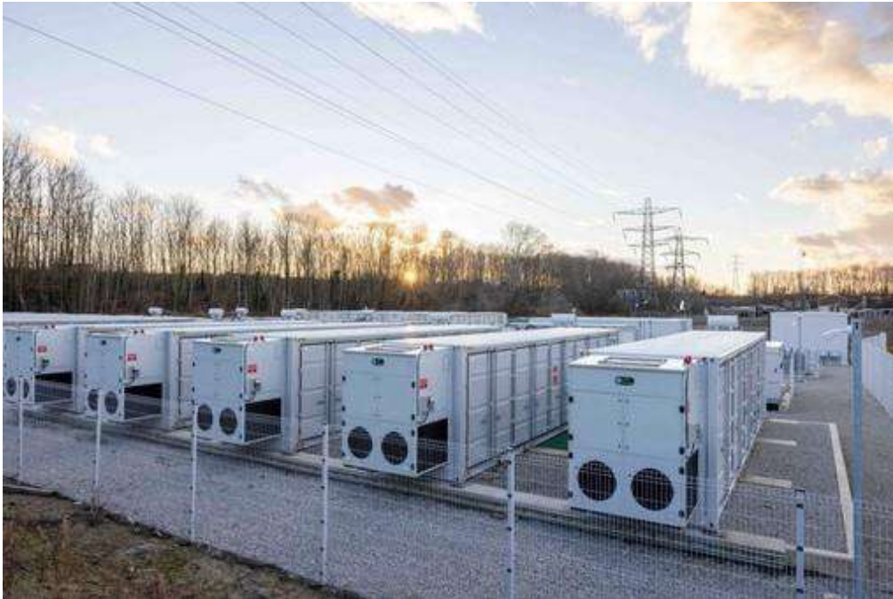
Figure 3-4: Example of a BESS Facility
