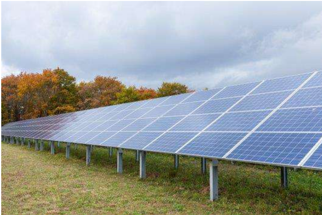
Figure 3-1: Example of a Solar Array
