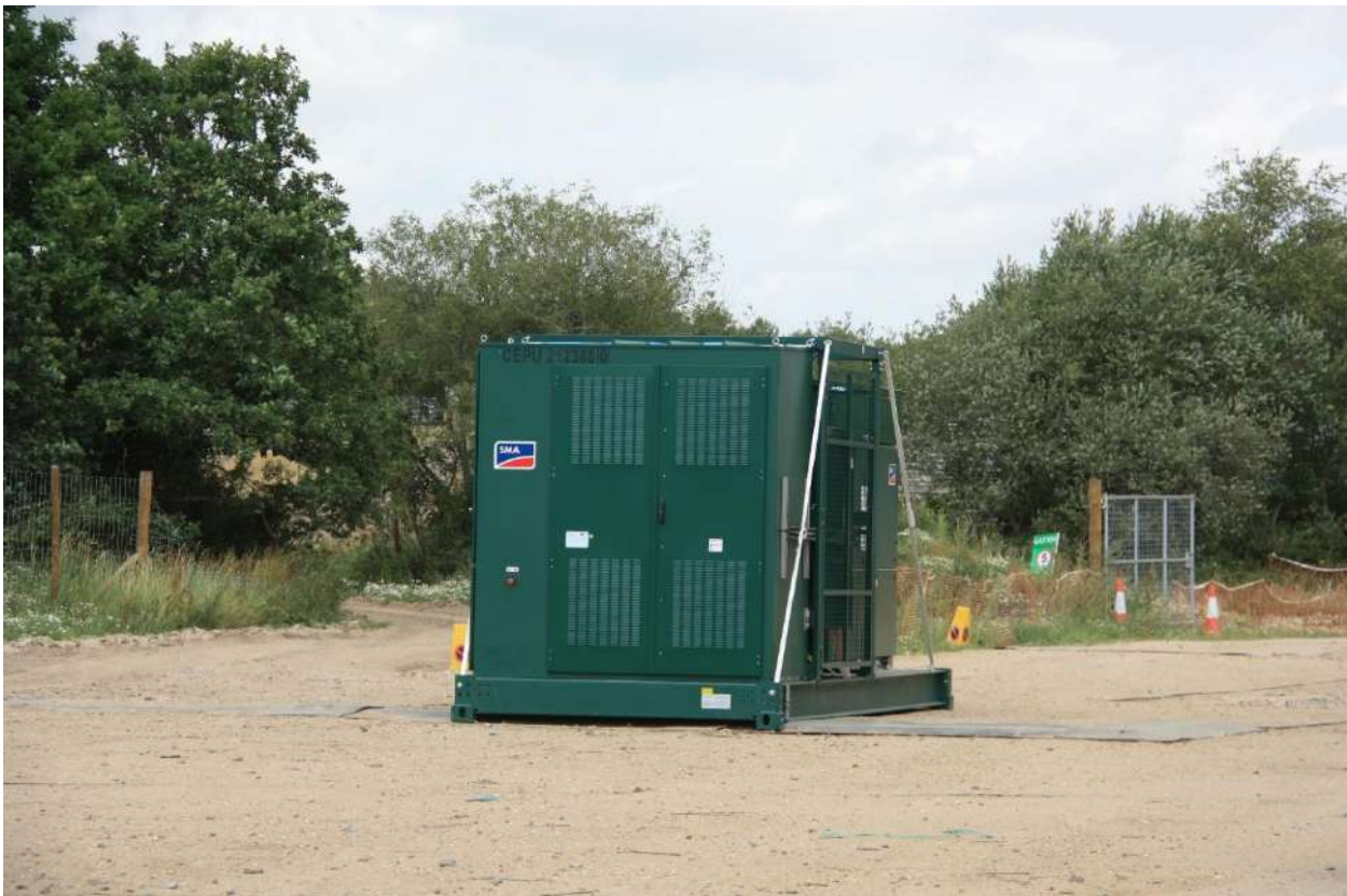
Figure 3-3: Example of a Central Inverter Container
