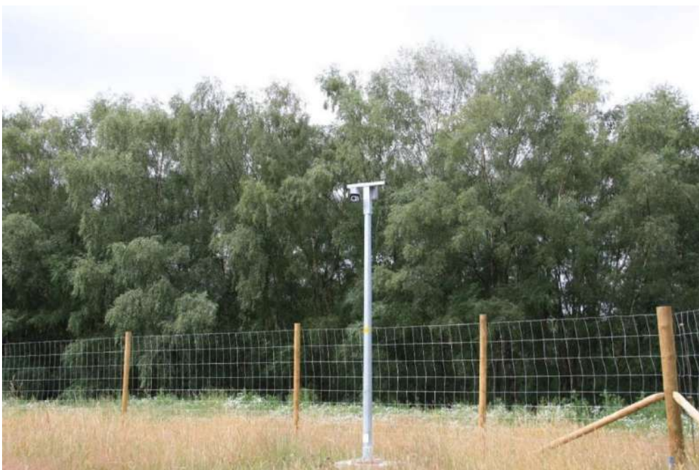
Figure 3-5: Example of Pole Mounted CCTV
